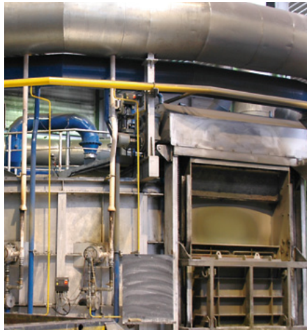
Rotary table furnace
