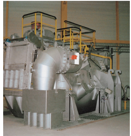
Aluminium tank furnace
