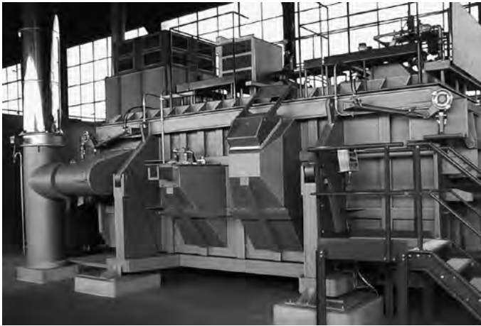
Aluminium industry: smelting furnace
