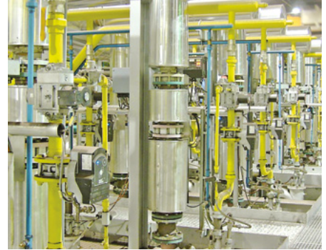
Walking beam furnace with overhead firing
